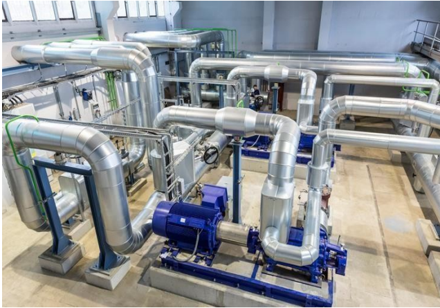
Industrial Piping System
